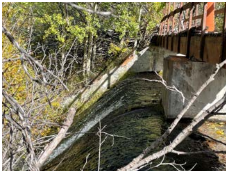
Downstream Side of Dam showing Spillway, Catwalk, Orange-Colored Pedestal, and Lifted Decking
